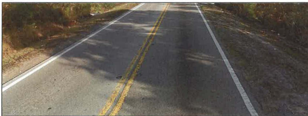
Figure 4- 1: Pavement Condition of Orange Avenue
