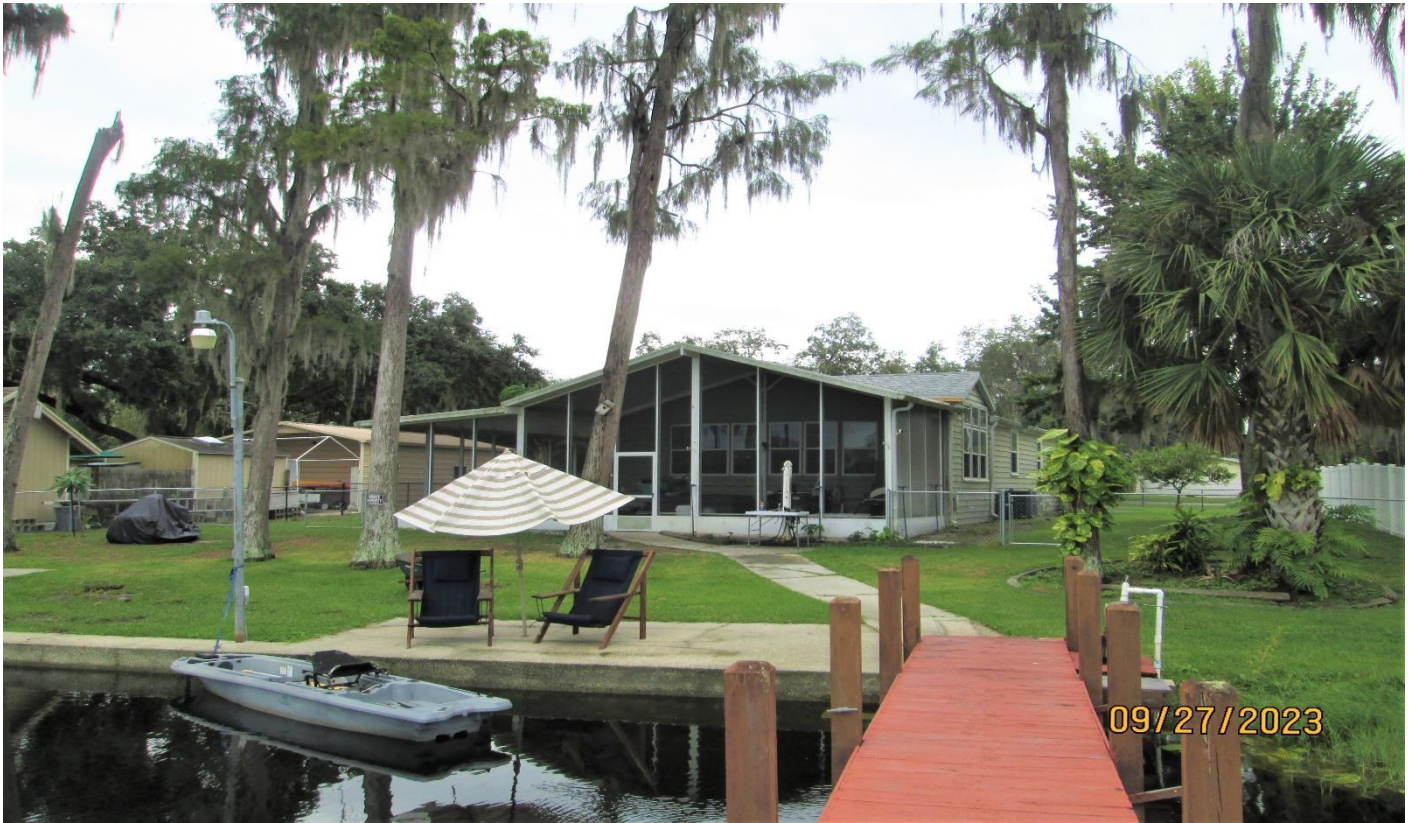
Boat dock, facing south towards portion of existing screen room encroaching in NHWE
