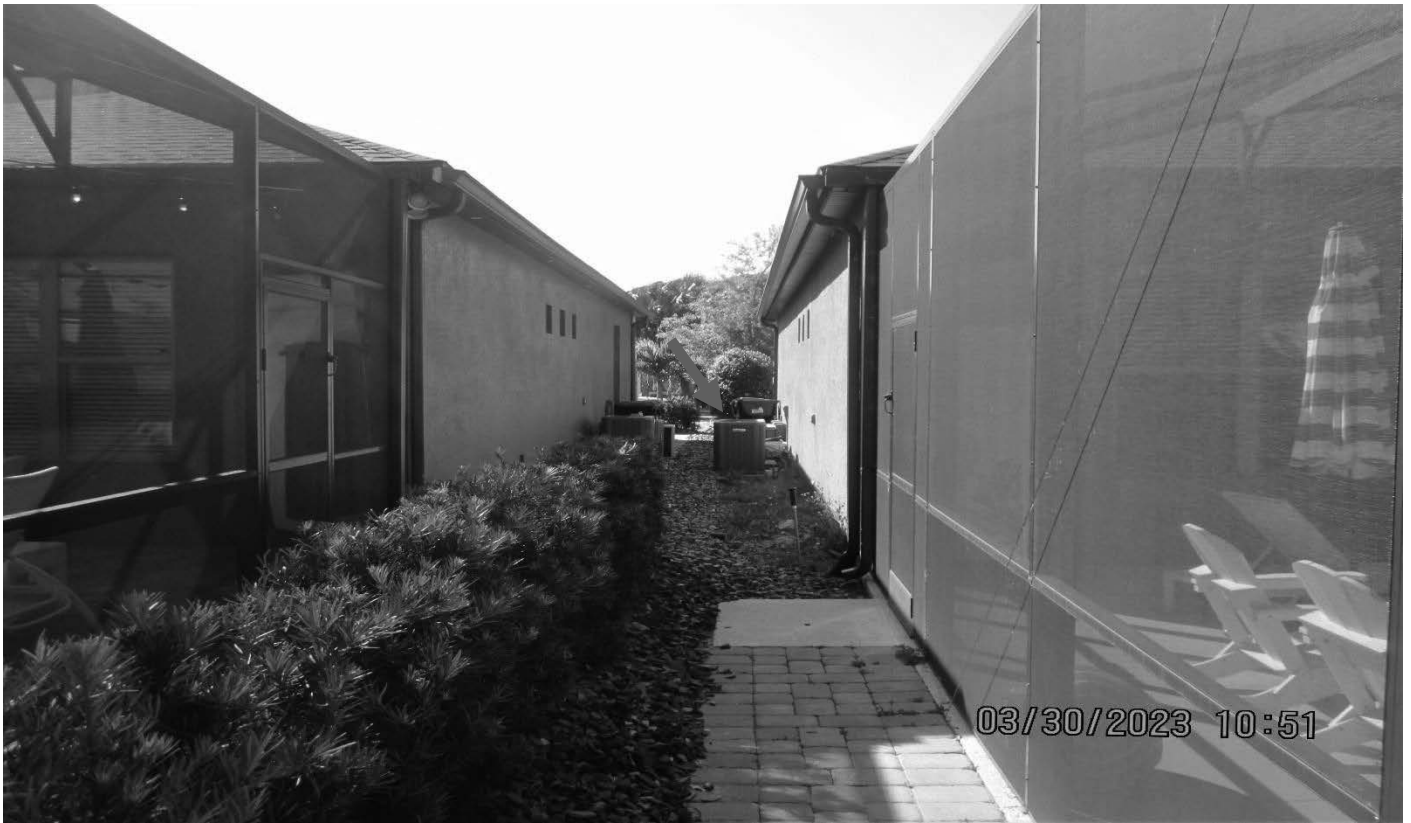
East side- Existing air conditioning unit, facing north
