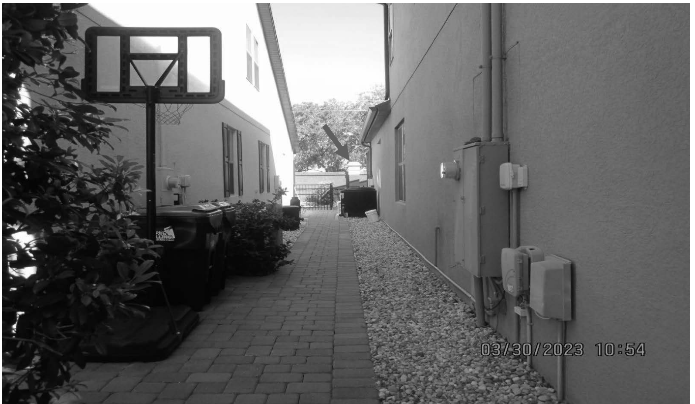
West side - Existing pool equipment location, facing north
