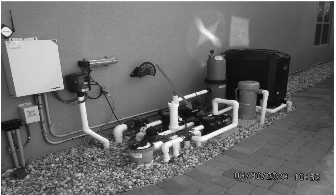
West side – Close up of existing pool equipment, facing southeast
