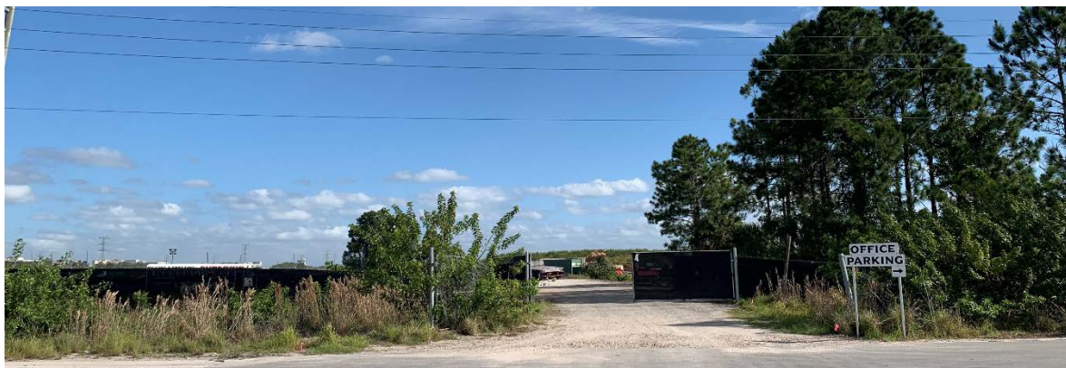
Site No. 29 – Universal City Property Management III LLC Site Reconnaissance: Construction activities
