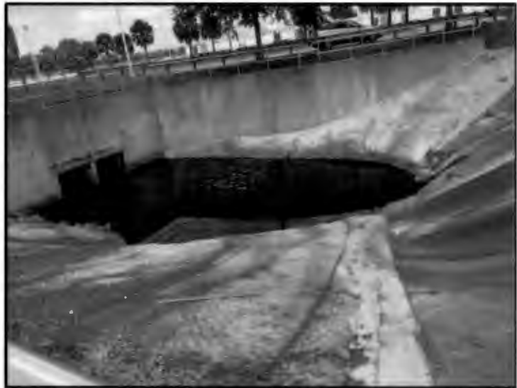
Upstream end of the 84-inch RCP culvert crossing (west of Tradeshow Boulevard).
