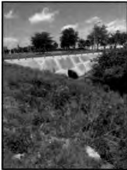
Downstream end of the 84-inch RCP culvert crossing (east of Tradeshow Boulevard).
