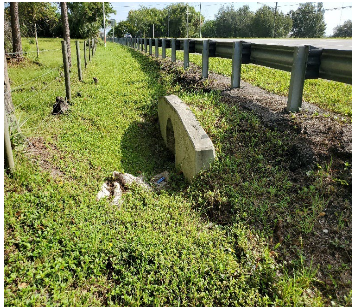
Cross drain which conveys runoff from basin 4-300 to storm drain on east side of Chuluota Road, facing north and east.
