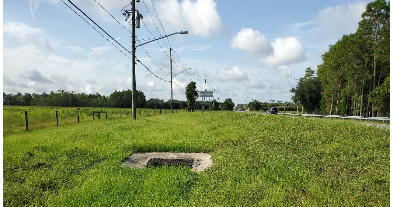
Ditch bottom inlet which conveys sheet flow from Chuluota Road to existing storm drain, facing south
