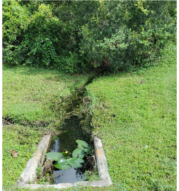
Existing side drain under Corner Lake Drive which conveys runoff from Basin 2B to Basin 3
