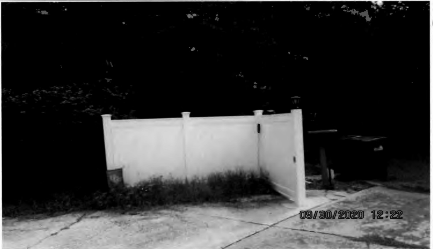
Section in violation in southeast corner of property looking east
