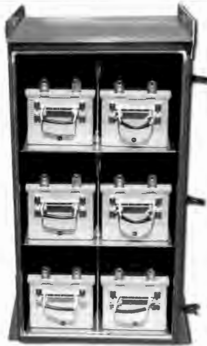
(6) Battery Bank : 8G8D
