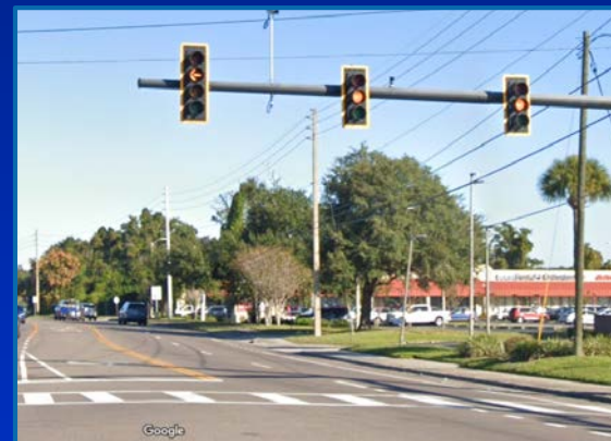
Flashing Yellow Left-turn Signal
