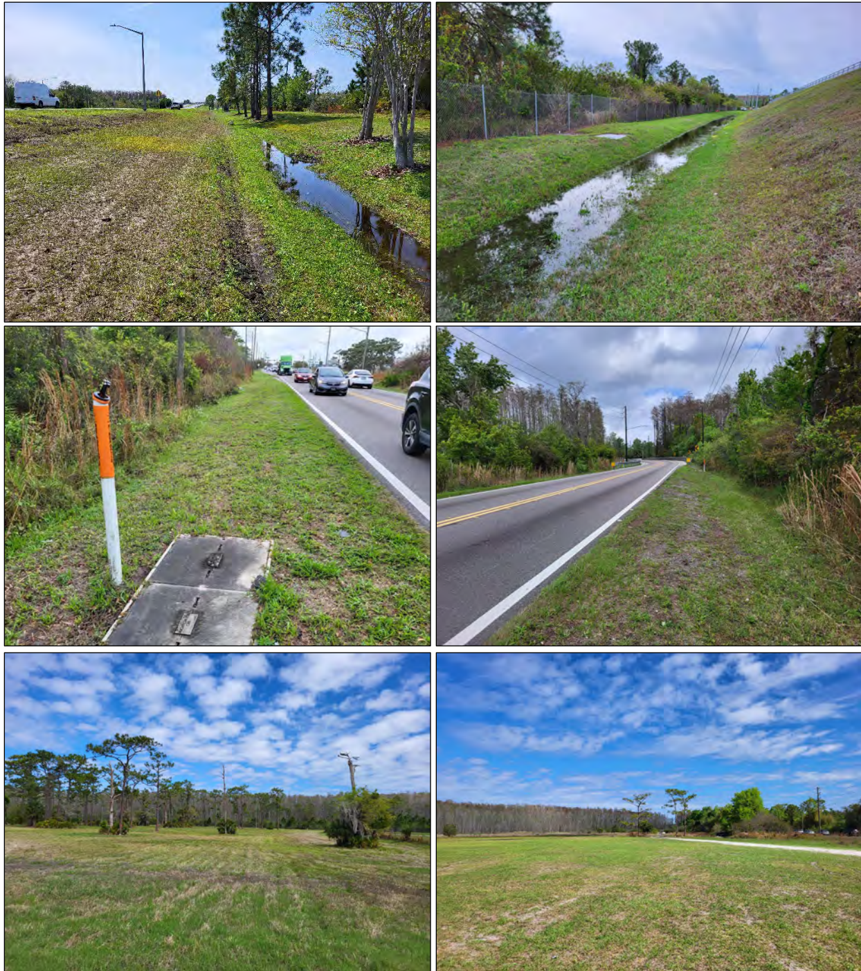
Figure 10. Overview of the archaeological APE. Top left: view south along the western side of Orange Avenue with roadway berm, inundated ditch, and utilities in northern portion of the APE. Top right: overview of utilities, inundated drainage ditch, and slope west of the Florida Turnpike overpass, view south. Center left: buried utilities and narrow ROW along the east side Orange Avenue in southern portion of the APE, view south. Center right: buried utilities along Orange Avenue in the central portion of the APE, view north. Bottom left: view north within westernmost pond footprint. Bottom right: view north within pond footprint immediately west of Orange Avenue.
