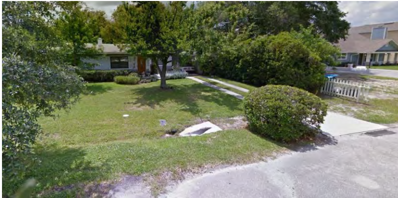
Drainage canal under driveway
