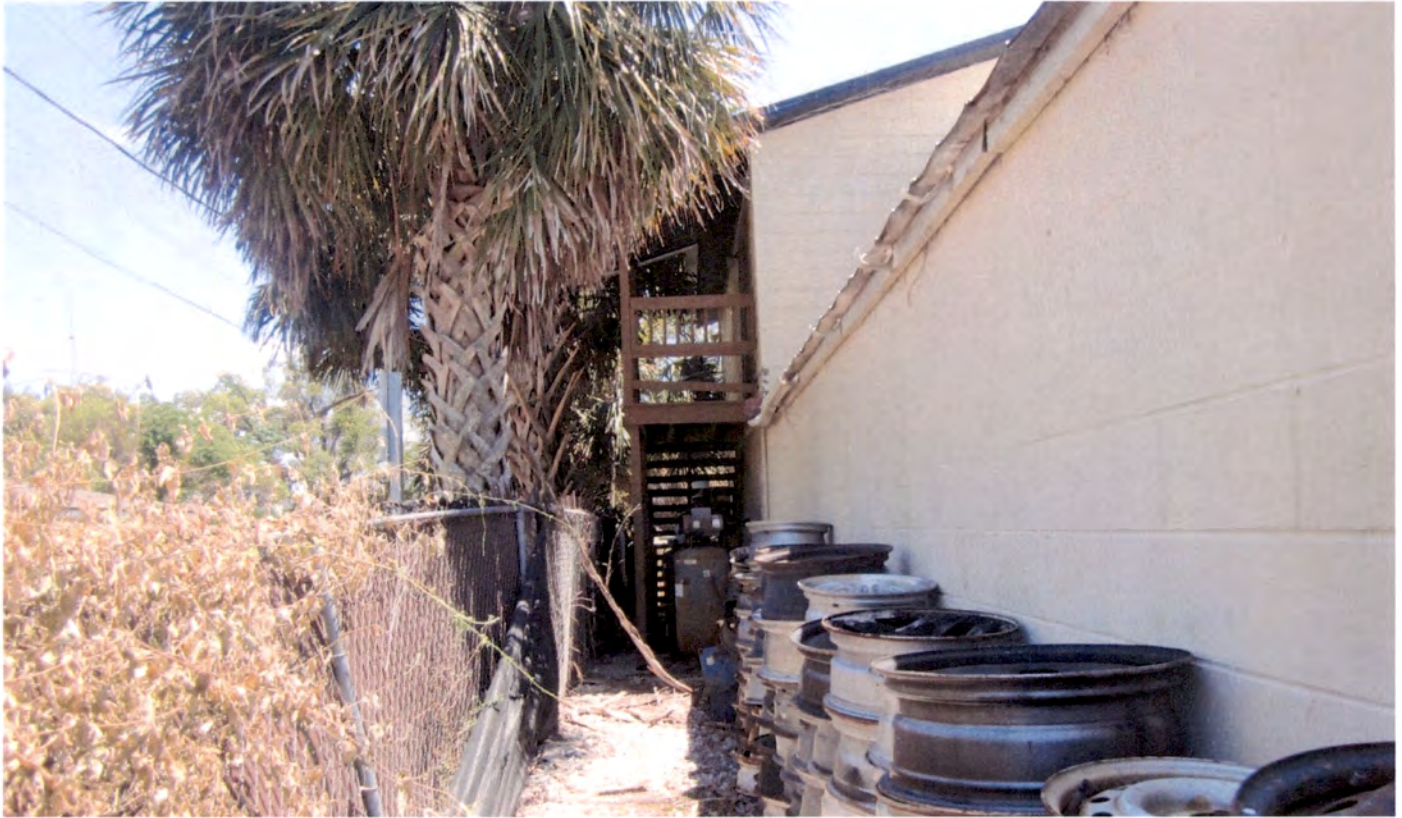
Rear of existing structure, facing south towards Variance #1 and alley (on left)
