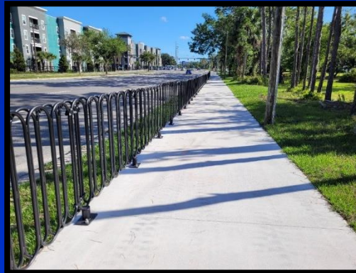
UCF - Fence installed along new 10 ft multipurpose path to channel pedestrians to cross safely at the signalized intersection
