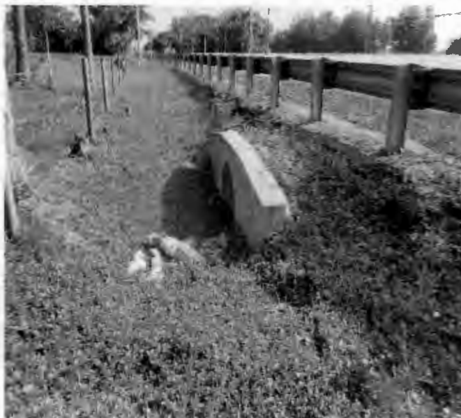
Cross drain which conveys runoff from basin 4-300 to storm drain on east side of Chuluota Road, facing north and east.
