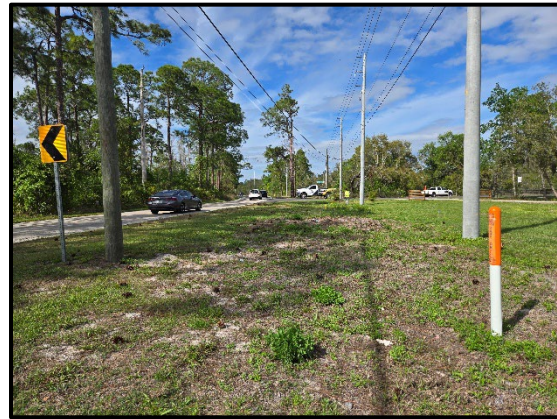
Photo 2.6. Utilities (powerlines, gas line, fiber optic) along the northbound side of Avalon Road, facing north.
