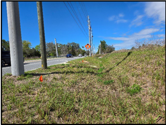
Photo 2.29. Drainage ditch between berm and powerline corridor adjacent northbound Avalon Road, facing north.
