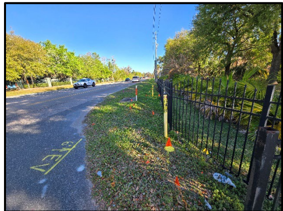
Photo 2.20. Private residential fence with clustered marked utilities along northbound Avalon Road, facing south.
