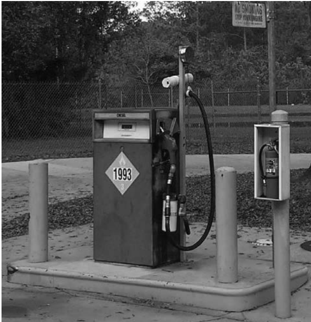
Fuel Pumps Installed in 1986 (33 years ago)
