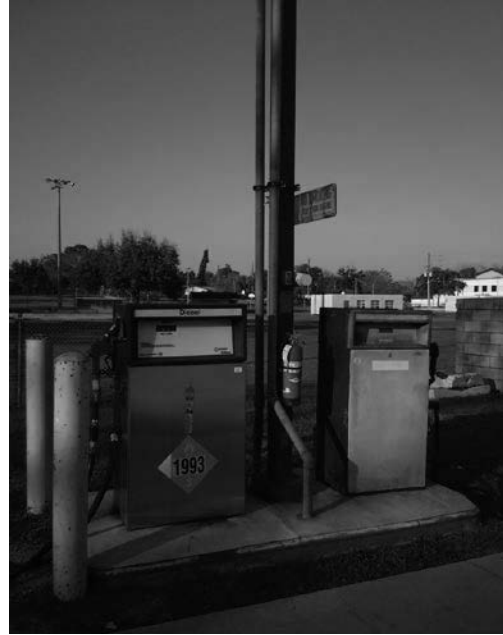
Fuel Pumps Installed in 1991 (28 years ago)
