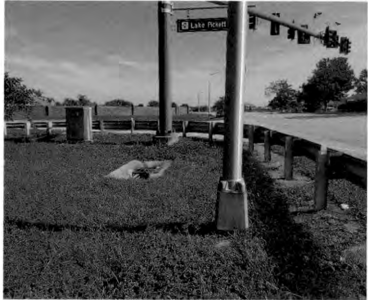
Ditch bottom inlet at southwest intersection of Lake Pickett Road and Chuluota Road, facing north
