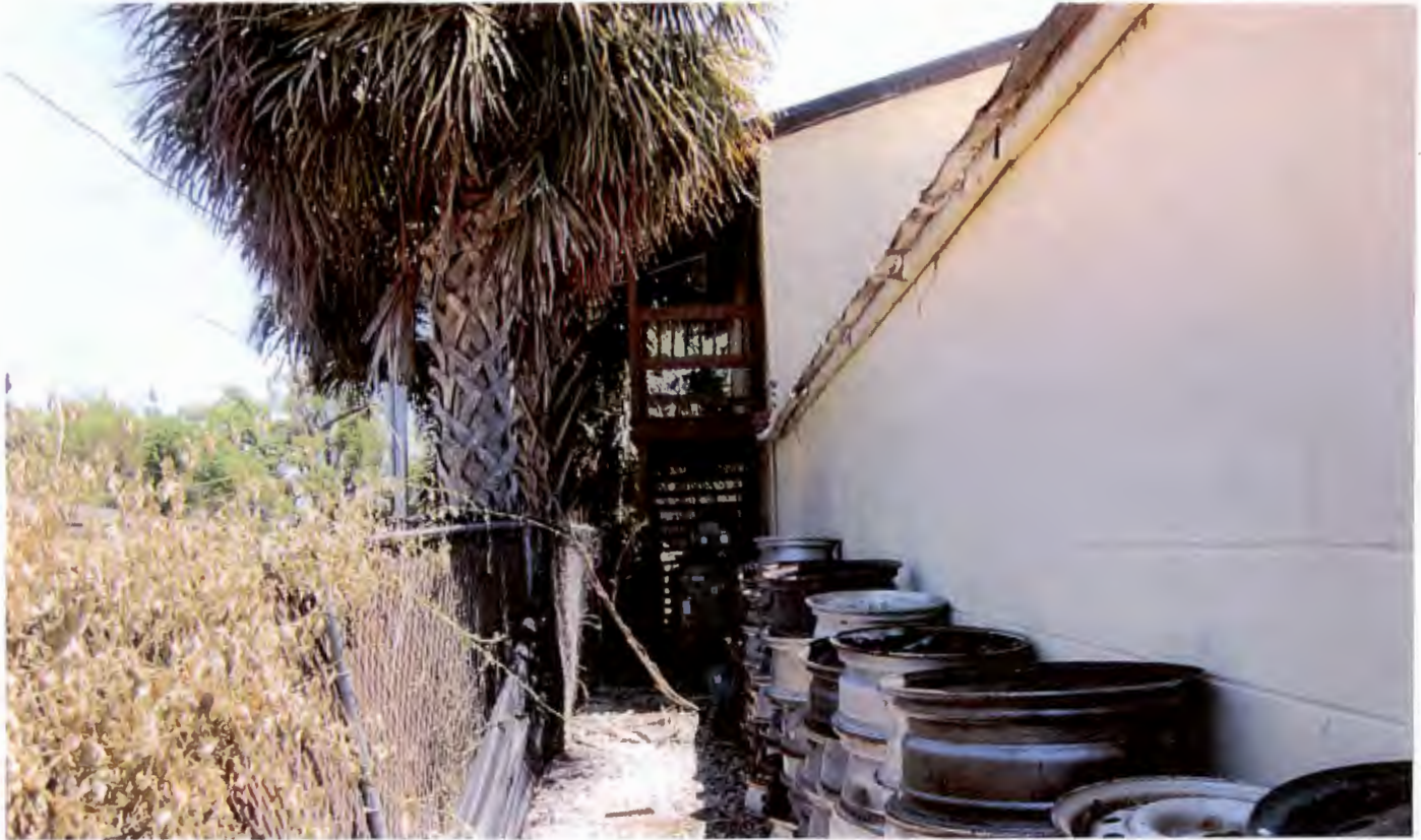
Rear of existing structure, facing south towards Variance #1 and alley (on left)
