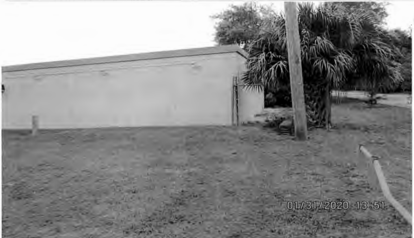
Variance #2; Bldg. G Existing 8.67 ft. Rear Setback in Lieu of 15 ft. Looking South
