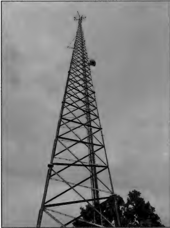
Figure 3 Top Half of Lattice Tower
