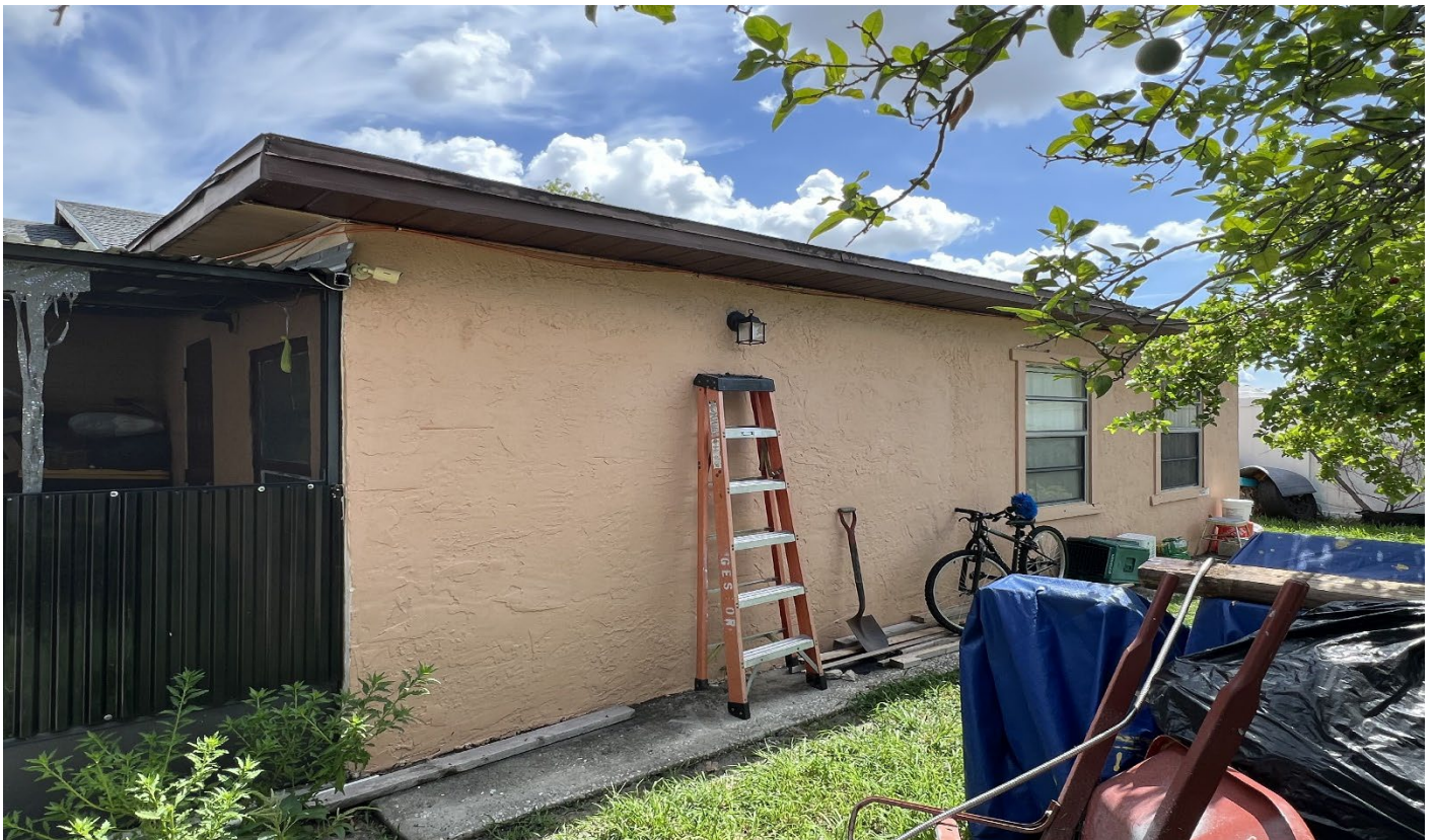
Rear yard, facing northeast towards the existing unpermitted addition and location of proposed addition
