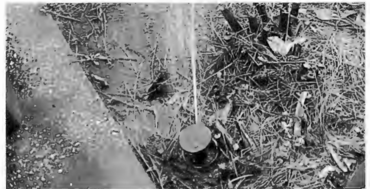
Figure 15. Object is interfering with spray pattern, resulting in poor distribution uniformity
