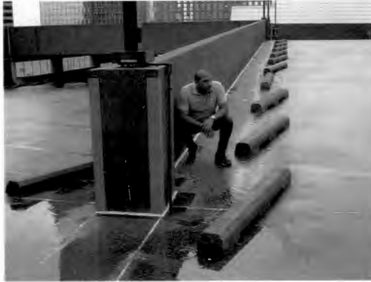
Parking Garage Hazard
