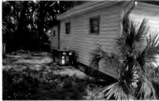
HVAC unit not elevated
