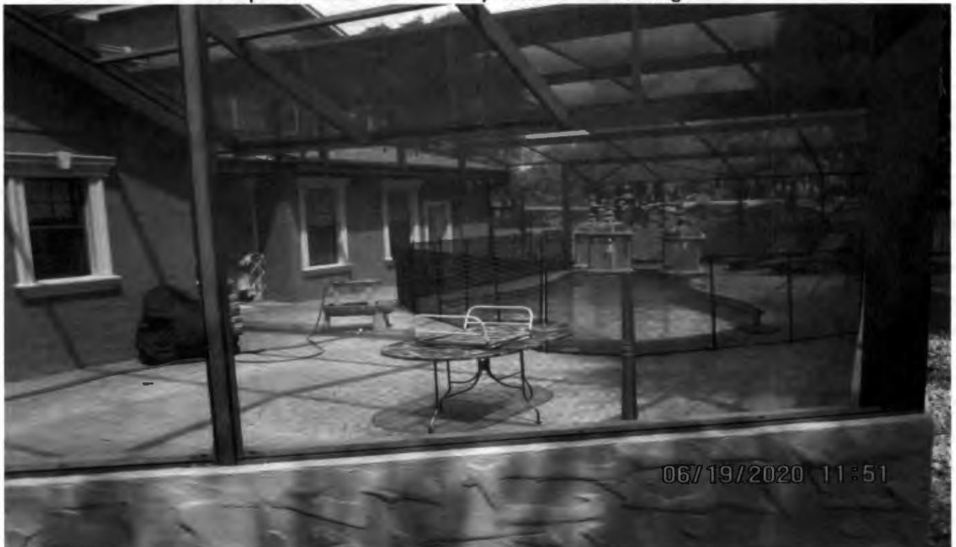
Portion of existing screen enclosure proposed to be converted to covered porch addition looking west
