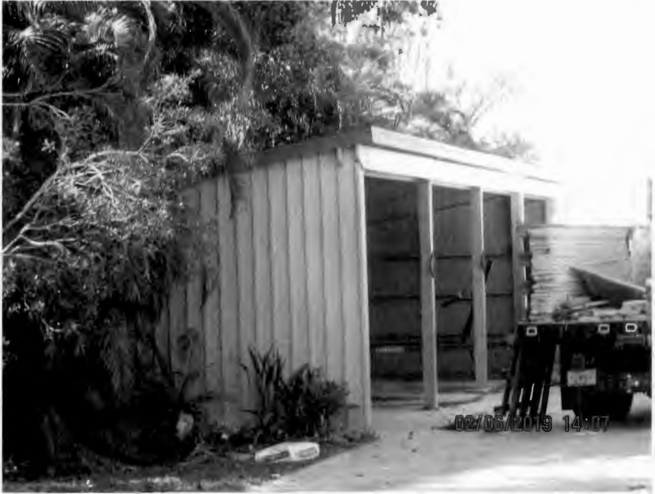
Existing Unpermitted Carport
