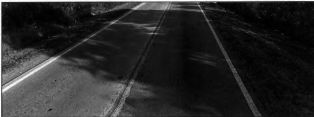
Figure 4- 1: Pavement Condition of Orange Avenue
