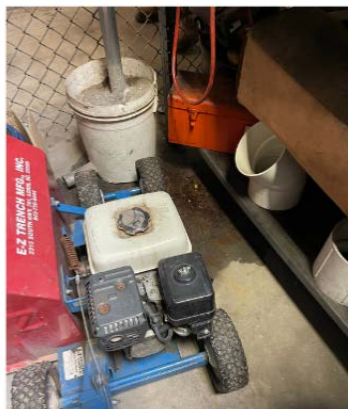
Gas or oil leak on Operations floor
