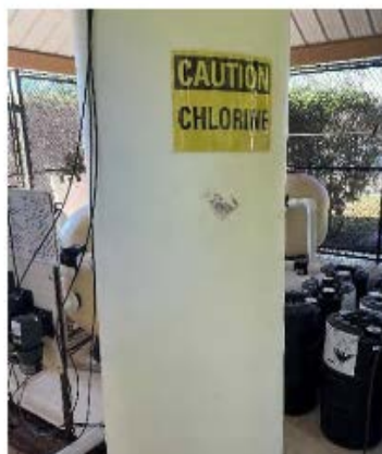
Chlorine stored with acid
