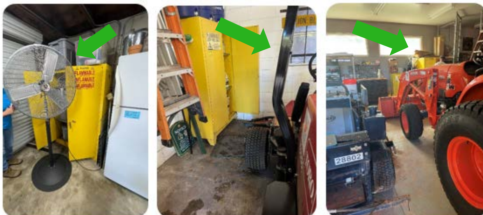
Combustible items on top of fire safety cabinets and obstructed access to cabinets
