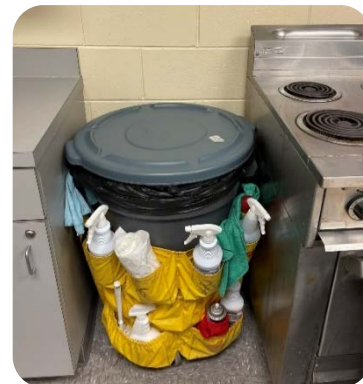
Flammable materials stored next to stove
