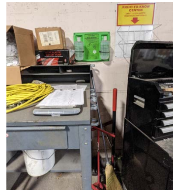
Eyewash station with obstructed access at Operations
