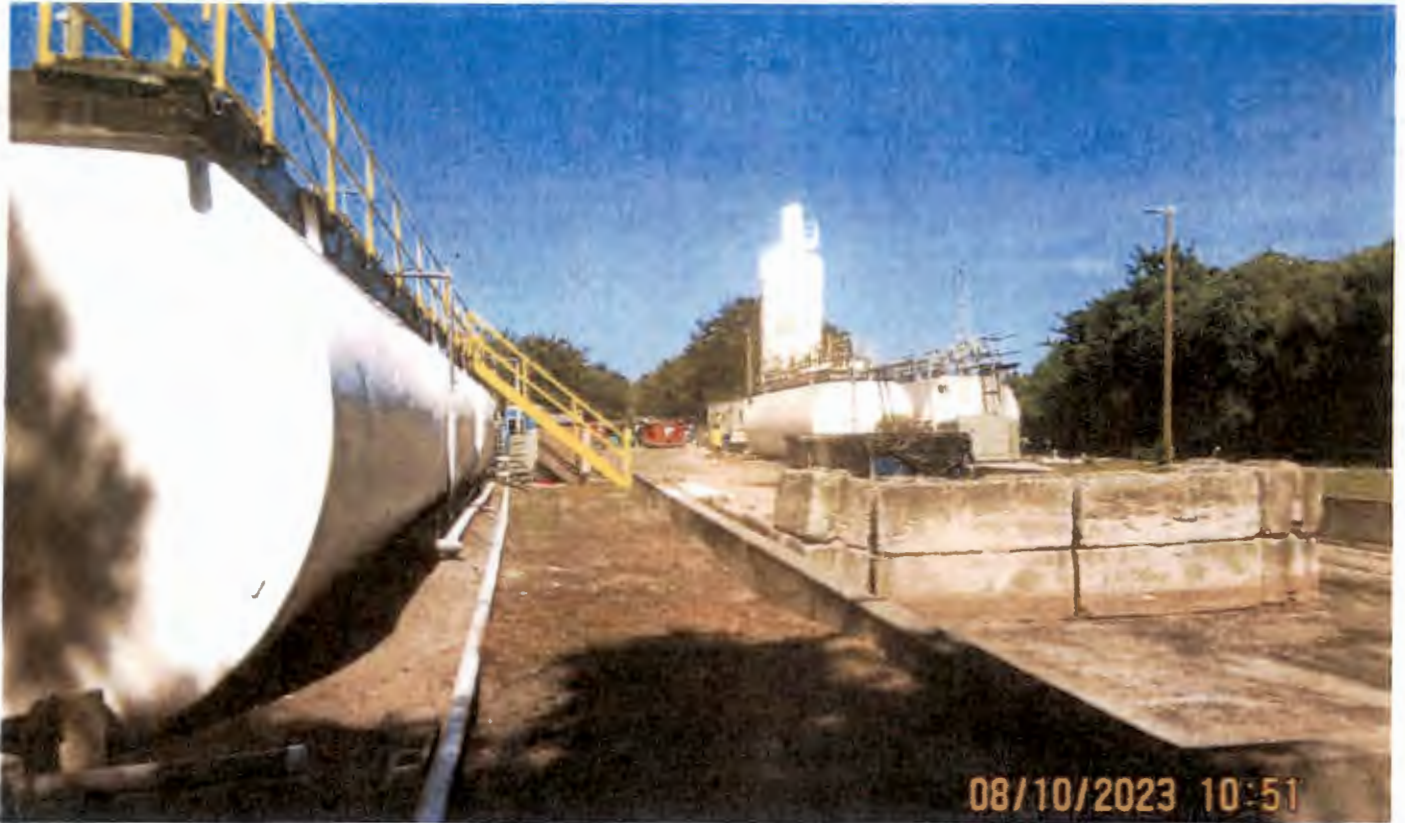
Near northeast corner of site facing northwest to silo, solids dewatering area, tanks - left & at rear
