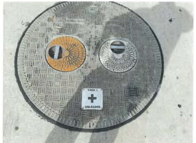
Tank 3 Unleaded Fill Sump
