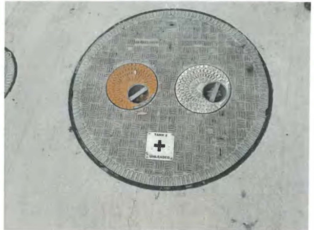
Tank 2 Unleaded Fill Sump
